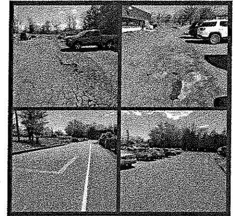
The parking lot at BARC Production Services Quakertown, saw a full renovation thanks to a grant from Bucks County Community Development.
